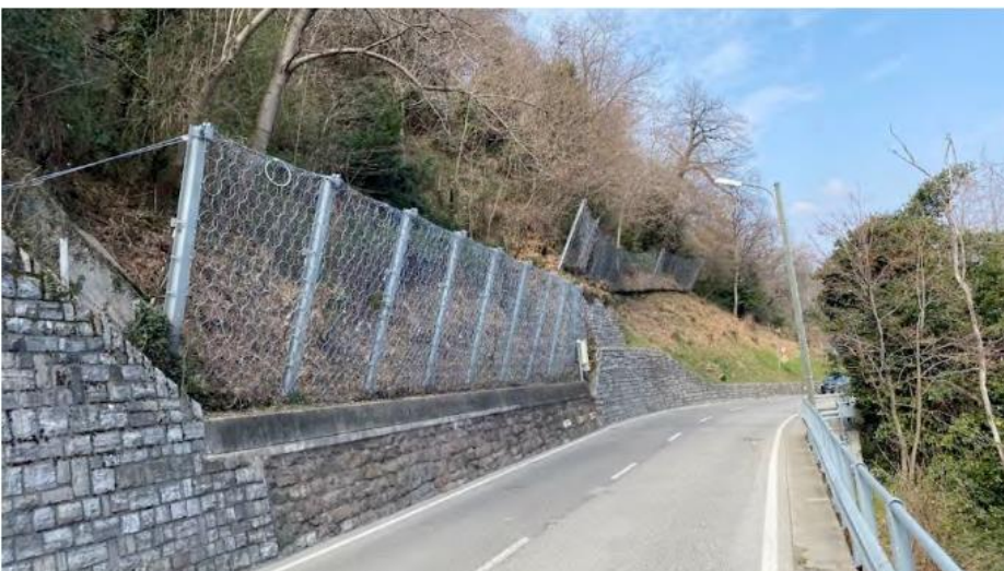
Rockfall attenuators protecting the road and preventing accidents. Photo courtesy of Michel Di Tommaso.
