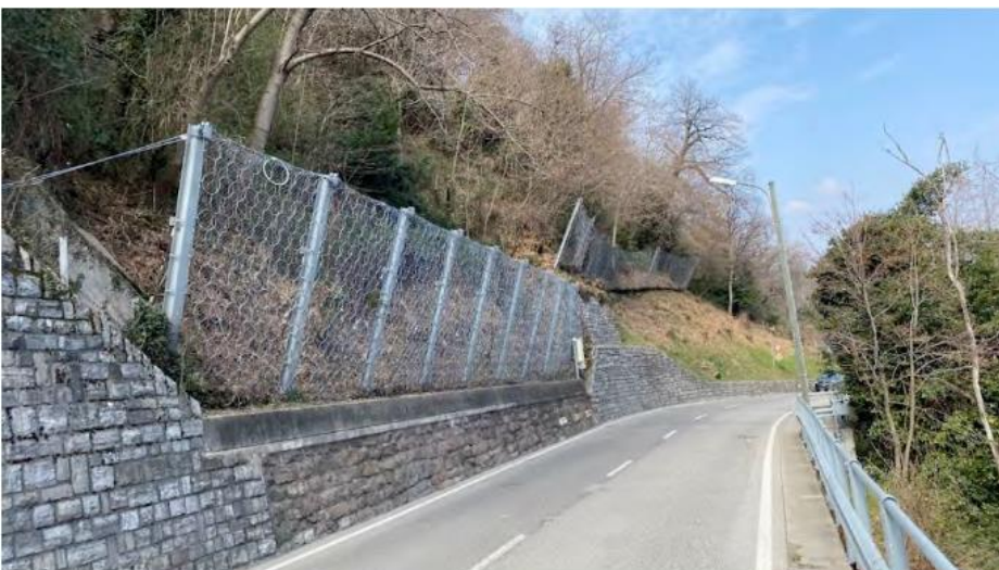
Rockfall attenuators protecting the road and preventing accidents. Photo courtesy of Michel Di Tommaso.
