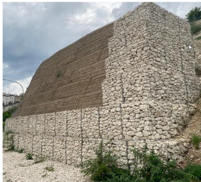
Gabion walls are used to control erosion. Photo courtesy of Michel Di Tommaso.
