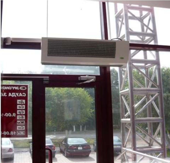
Air curtains at the entrance
