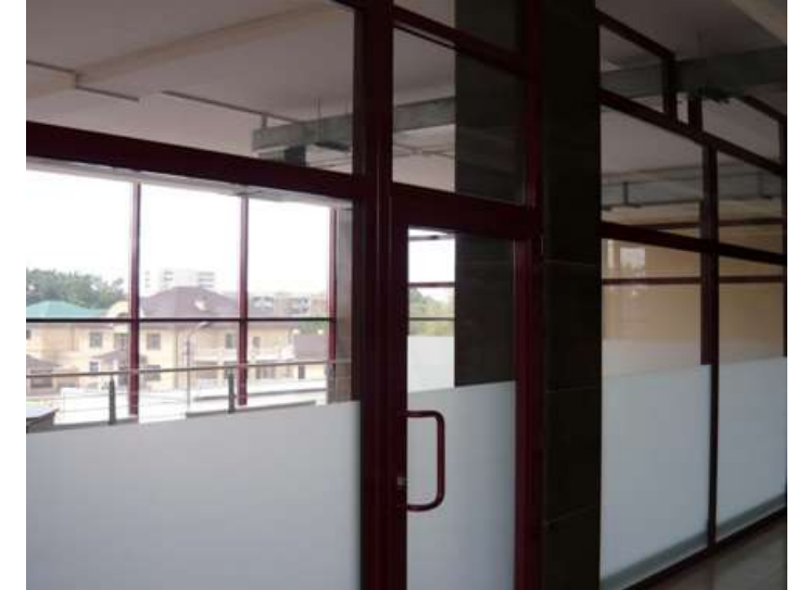
Precise separation of cold and warm zones using aluminium partition walls (stairwells/office areas) AS A RESULT: NO DRAUGHTS
