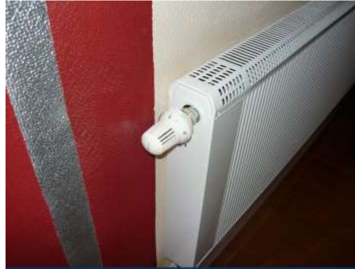
Copper-aluminium radiators with built-in Danfoss thermostatic valves and low heat inertia (10 times less than cast iron radiators - 15% of the heat load) are used.
